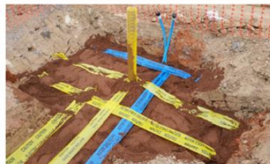
2. Vertical sleeves placed to protect any purge valves (nipples). Loaded with sand and marker tape
