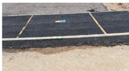
7. Completed Stage 1 footpath with pit ready to be excavated at stage 2 (future connections)
