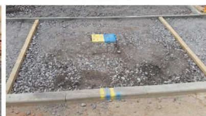
6. Preparing for future gas and water connections with timber bearers and sprayed brick over vertical sleeve
